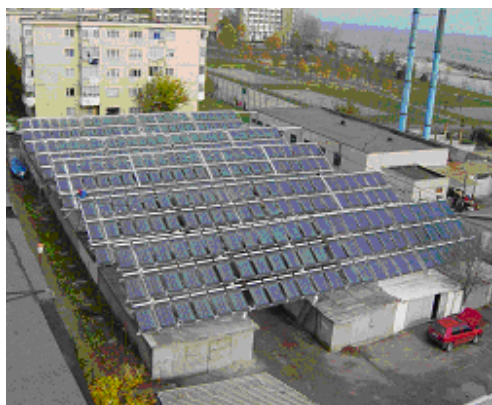
Fig. 4 Solar thermal system in Mangalia city
