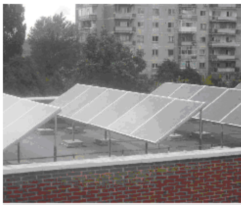
Fig. 5 PV plant on the Polytechnic University Bucharest
