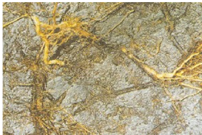
Fig. 1 Roots leaving impression on waterproofing membrane, adapted [10]
