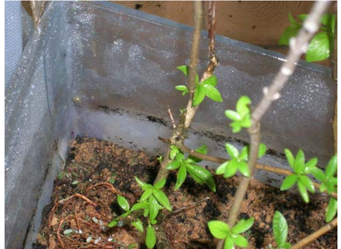
Fig. 11 Growth observed between joints of the membranes
