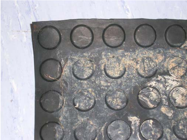
Fig. 9 Clean sheet membrane edges indicate no form of growth between the liquid applied waterproofing and sheet membrane
