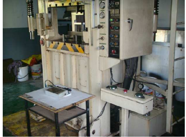
Fig. 7 Installation of the device for oil pressure measurement to the hydraulic press
