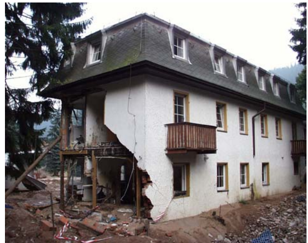
Fig. 1. Example of a close to collapse building with intact floor parts. Photo: Michael Markus.
