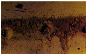
Fig. 2 Ductile iron pipe corrosion
