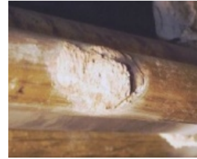
Fig. 6 Galvanic ringworm corrosion
