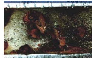
Fig. 7 Corrosion of galvanized potable water piping
