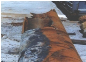
Fig. 1 Ductile iron pipe failure
