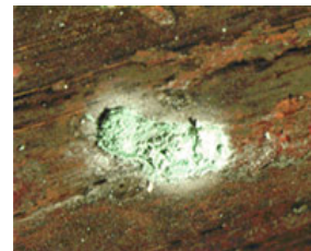
Fig. 8 Pitting corrosion of copper pipes
