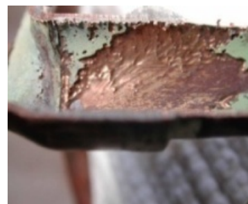
Fig. 10 Copper pipe corrosion
