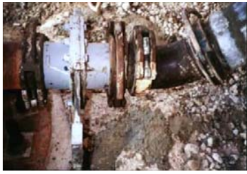
Fig. 12 Corroded metallic fittings of pipelines removed for replacement
